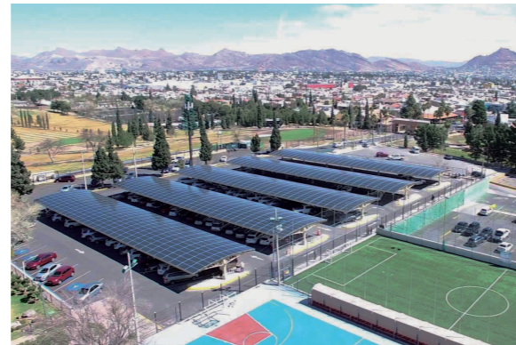
MEXICO CITY, MEXICO 1MWp Module Type: LR6-72 340Wp Completion Date: Mar. 2018
