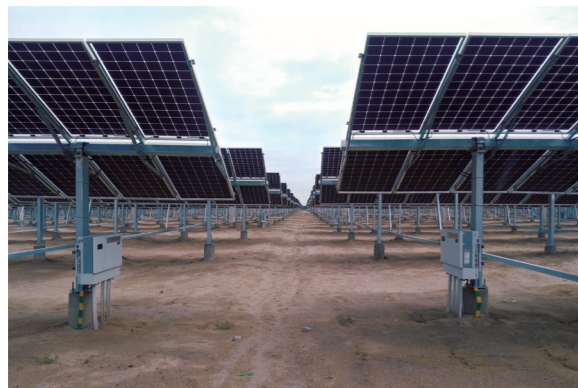
GOLMUD, QINGHAI, CHINA 20MWp Module Type: LR6-72BP 350Wp Completion Date: Dec. 2017
